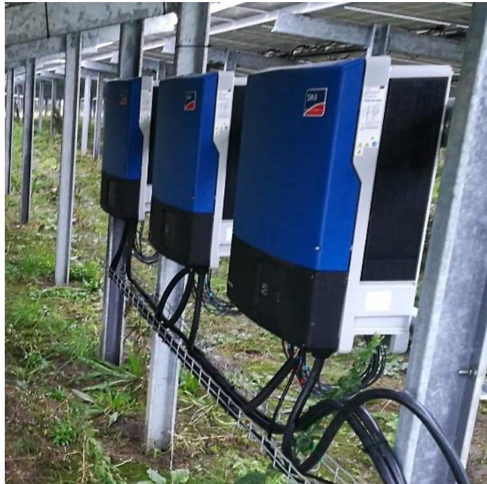
Photo 3 Example string inverters
