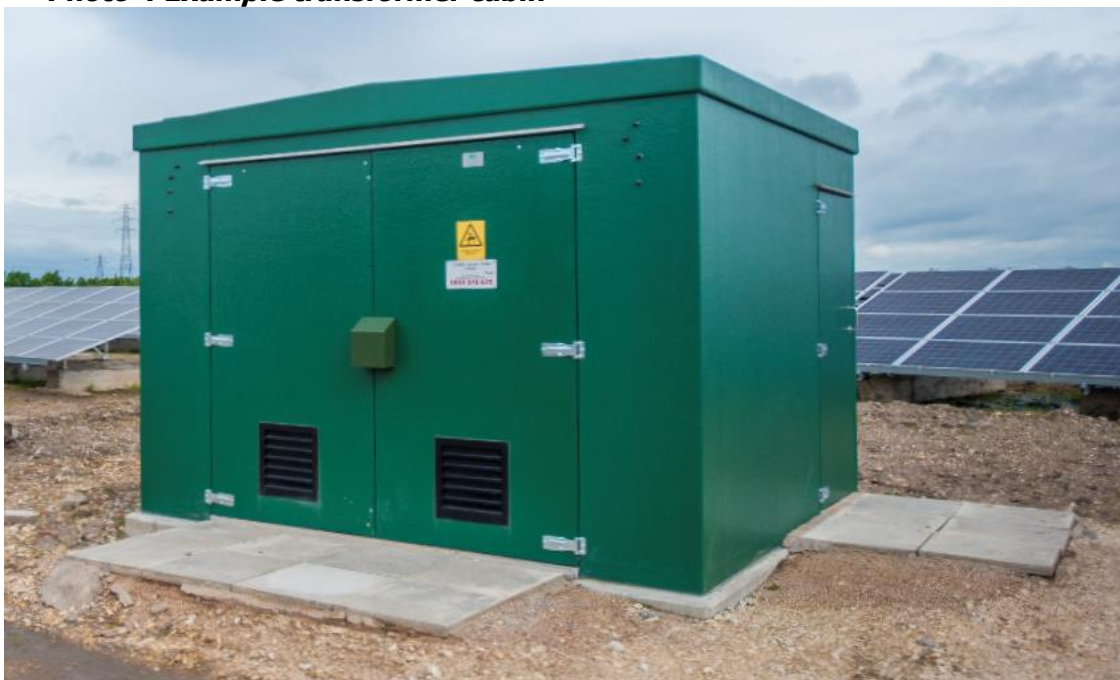
Photo 4 Example transformer cabin
